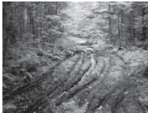
Damage to the Chubb Pond Trail in the Black River Wild Forest caused by illegal ATV use.
